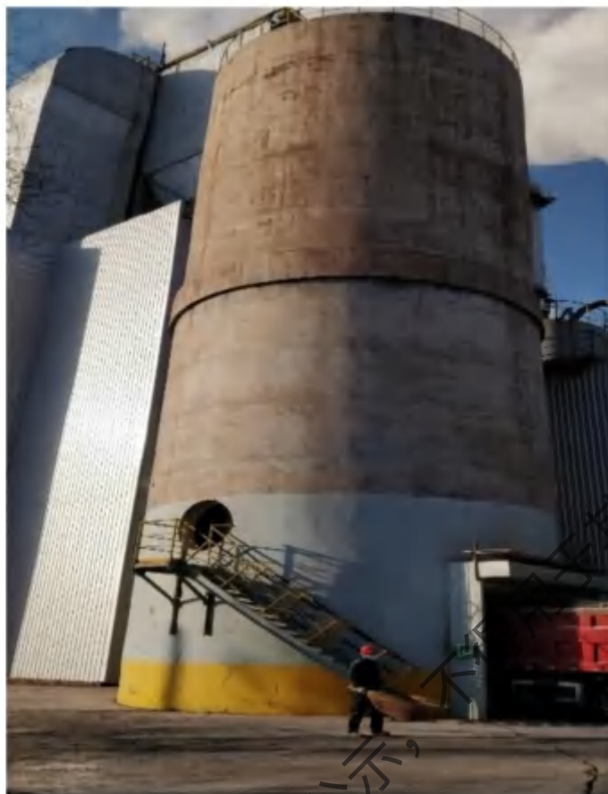
脱硫石膏筒仓
