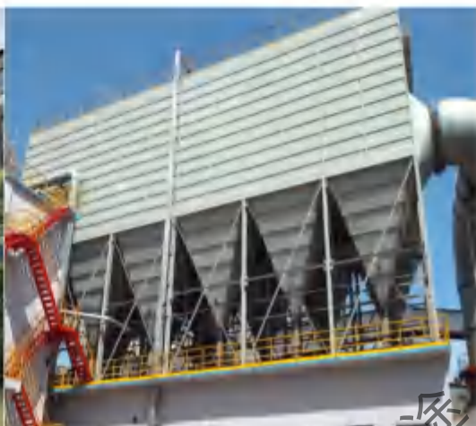
烧结成品储矿仓除尘
